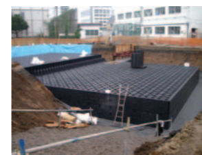
Rainwater storage facility under a schoolyard
