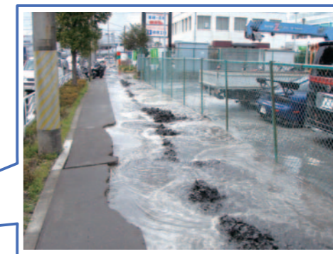
Liquefaction in the low-lying area caused by the Great East Japan Earthquake (March 11, 2011) • Sand and groundwater is gushing out of the crack in the road.
