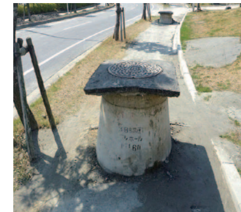
Manhole uplift due to liquefaction (Great East Japan Earthquake (March 11, 2011))
