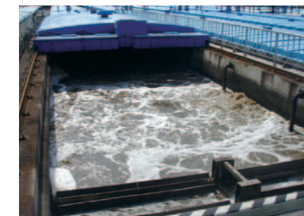
Example of reaction tank
