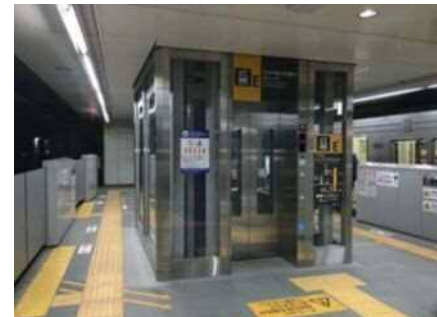
Elevator (Tokyu Shibuya Station)
